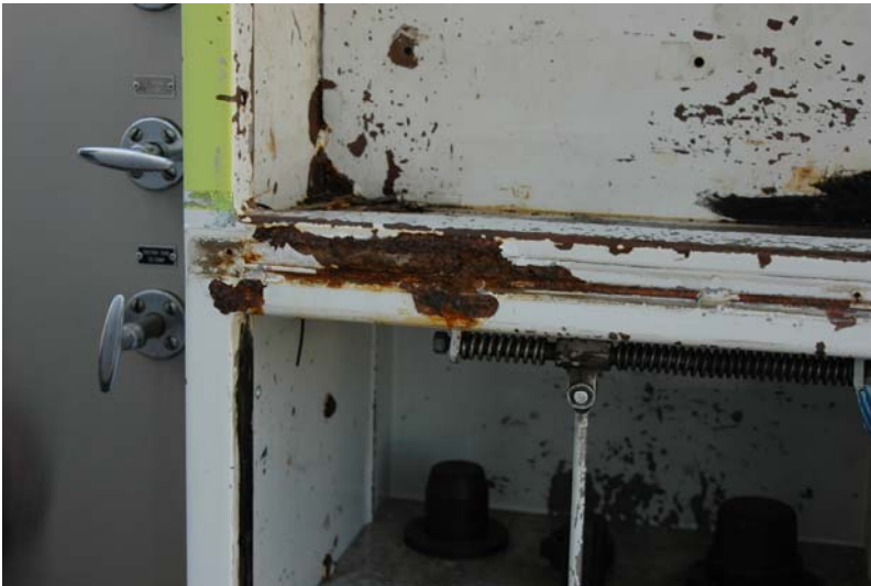
Dividing Rail (rust damage)
