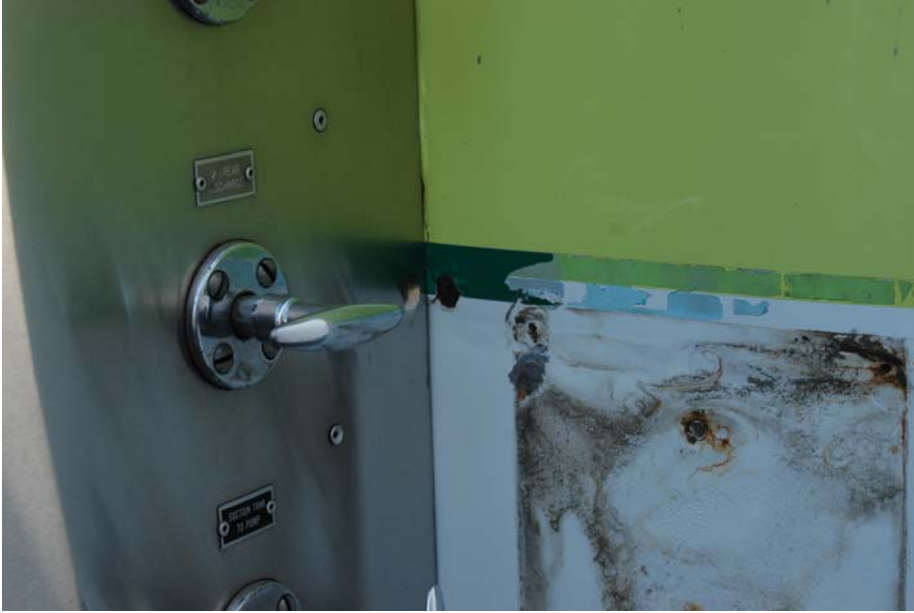
Front cabinet damage.
